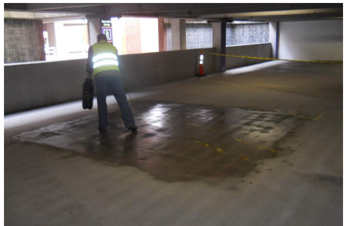
Fig. 8: Application of surface-applied corrosion inhibitor to parking garage surface at test area showing sectioned installation for ensuring adequate coverage rates
