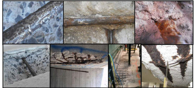
Fig. 3: Corrosion-related distress: (a) pitting from chloride-induced corrosion (after bar cleaning), (b) corrosion products compared to bare steel, (c) corrosion-induced cracking, (d) cross-section of delamination, (e) overhead delamination and spalling hazard, (f) horizontal spalling and tripping hazard, and (g) reinforcing steel disintegration
