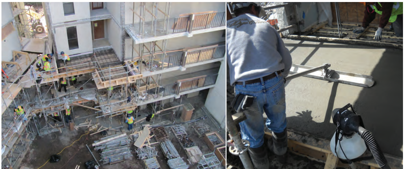
Fig. 8: Illustration of replacement of portion of walkway slabs (left) and balcony (right). Note the fogger at right of craftsman, used after finishing and prior to implementation of wet burlap and plastic for moist curing and insulating blankets when necessary
