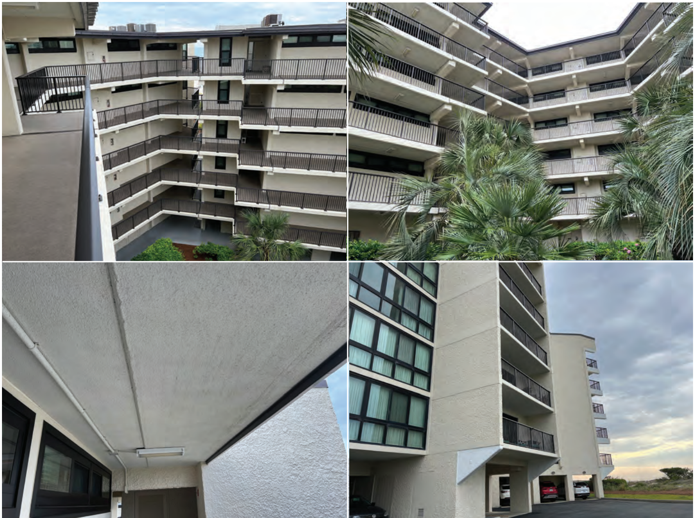
Fig. 13: Examples of current conditions: walkways (top left and right), soffit with thermal spray and coatings (bottom left) and replaced balconies with thermally sprayed haunches (bottom right)
