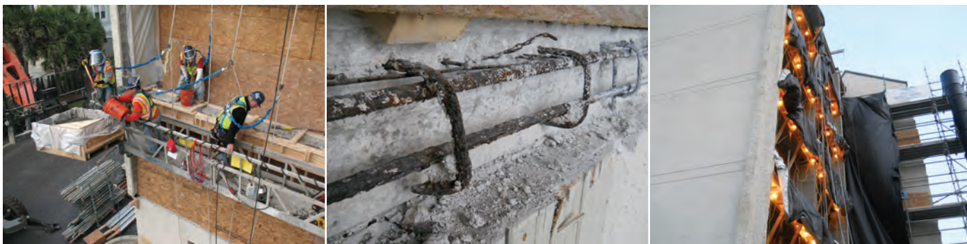
Fig. 5: Replacement of balcony slab edges from swing stage (left), example of corrosion of reinforcing steel during demolition (center), and example of thermal control (right)
