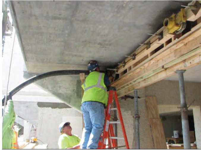
Fig. 12: Installation of self-consolidating concrete at a beam under a slab by pumping
