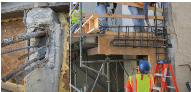
Fig. 9: Walkway cantilever beam showing removed concrete, low cover to bottom of beam, excessive cover to top tension reinforcing steel, and voids (top left), partially formed reinforcing steel for reconstructed beams and pilasters used to reduce the stresses in the beam (top right), and completed pilasters and beams cast integrally with the new concrete slabs (bottom). The pilaster was tied to the wall. Note the mechanical splices used to tie to existing steel for this beam.
